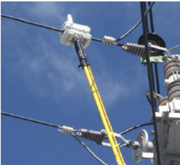
Fig. 38: Sensor installed using Grip-All hot stick
