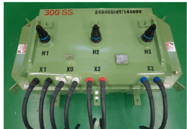
Fig.8 of paper 62: “SIDT” 3-ph 300kVA transformer
