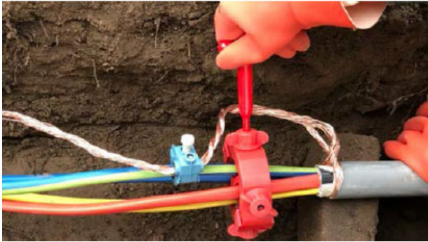
Fig. 8 of paper 1056: Screwing contact of short circuit ring through core insulation to secure operation on LV grid with PV installations
