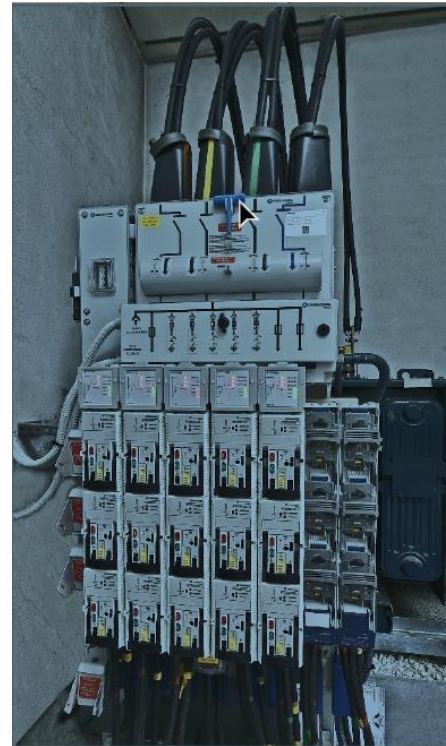
Fig 3 of paper 10713 : Automated LV switchboard
