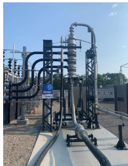
Fig. 4 of paper 11045: Photo of vertical Termination of superconducting 12kV cable - 62 MVA installed in Chicago in 2021 to increase the network
