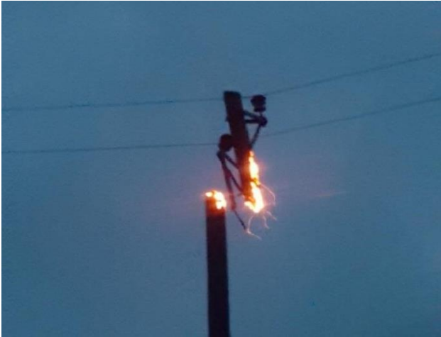
Fig. 1 of paper 10642 : Pole top burning in an advanced stage due to earth leakage current
