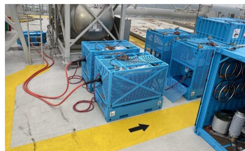
Fig. 4 of paper 11027: Setup of RTS at offshore substation
