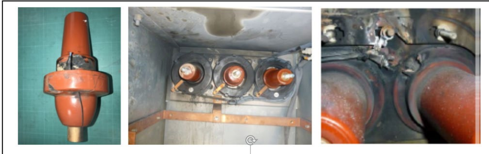
Figure 19 Practical examples of solid insulation failures
