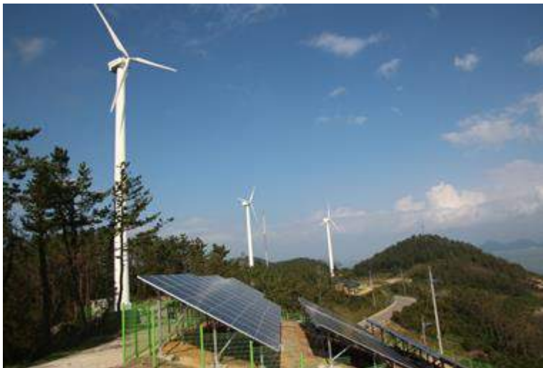
<Renewable energy complex of Gasa energy self sufficient island>
