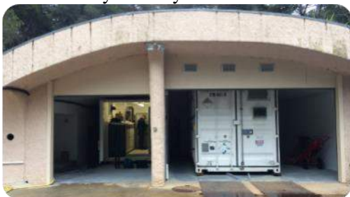
DSO battery (Grid Forming Unit)
