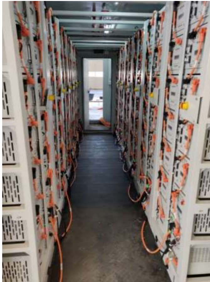
Figure 3.3-25: N470 Distributed batteries system.
