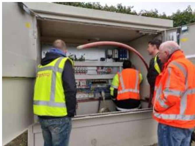
Figure 3.3-26: N470 Outdoor substation.
