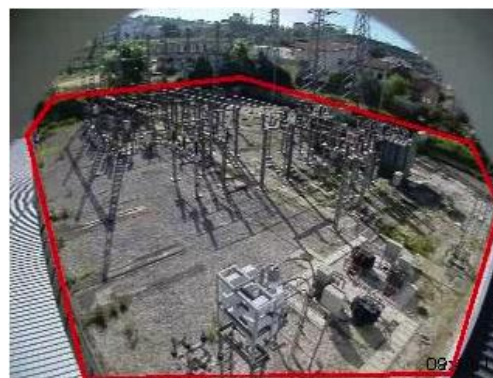
Figure 28 - Smart monitoring of substations
