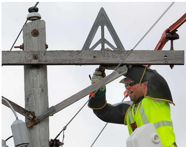
Figure 24 - Triangular pieces of plastic designed to stop large birds from perching along a stretch of power lines where an eagle was electrocuted earlier. (Iowa Source Media Group, Cedar Rapids, Iowa).
