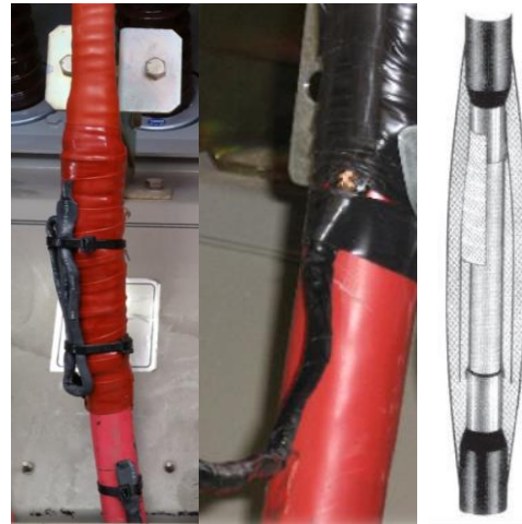
Figure 1 - Possible connection of the cable's shields. From left: 1) disconnected – 2) connected – 3) with insulation joint
