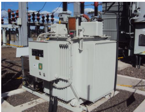
Fig. 10. ASC installed in Novo Hamburgo Substation – RGE Sul
