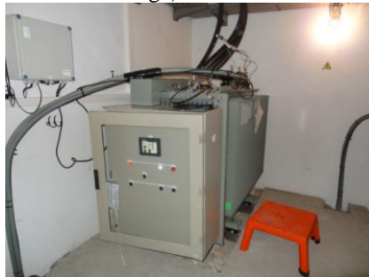
Figure 3 : installed OLTC picture
