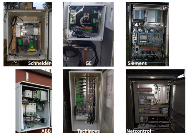
Figure 5 Example of RTU installations
