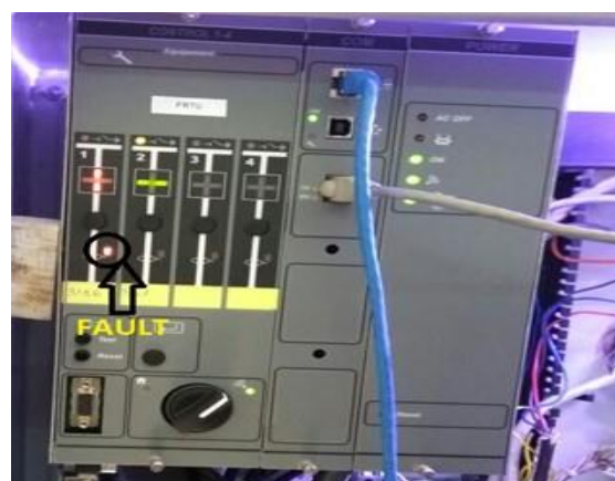
Fig:-4 Testing of Fault
