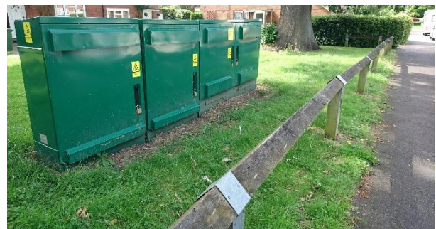
Figure 1 ESMU with one PEU (on the right) and two ESUs (on the left) installed on a grass verge near a footpath in residential area in Bracknell, UK.
