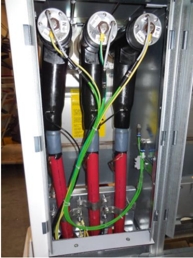
Figure 8 – LPVT sensors on RM6 Schneider-electric
