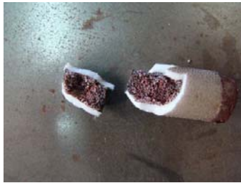
Figure 5, Fuse operation outside of its operation range.
