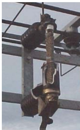
Figure 7, On-field low current operation failure due to aging.
