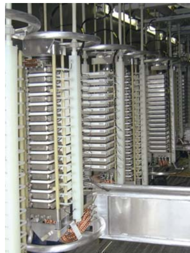
Fig. 8: SVC Light® valve assembly.
