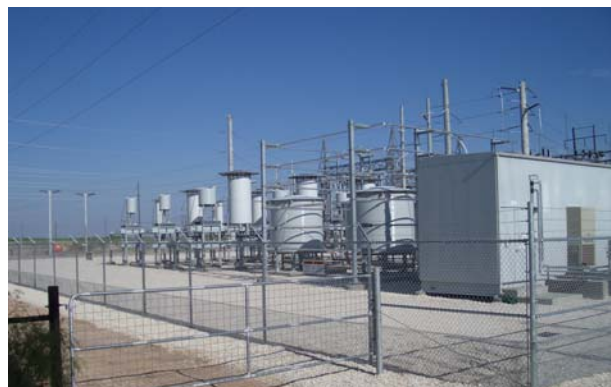
Fig. 5: Crane 69 kV, -40/+50 Mvar SVC, Texas.
