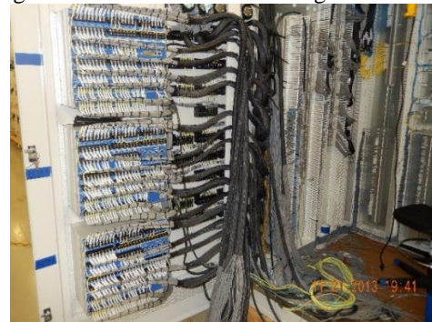
Figure 1 A data center low voltage compartment example showing conventional CT wiring for a bus differential
