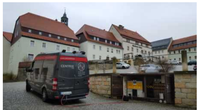
Figure 4: Connection of PD diagnostic system to the test object
