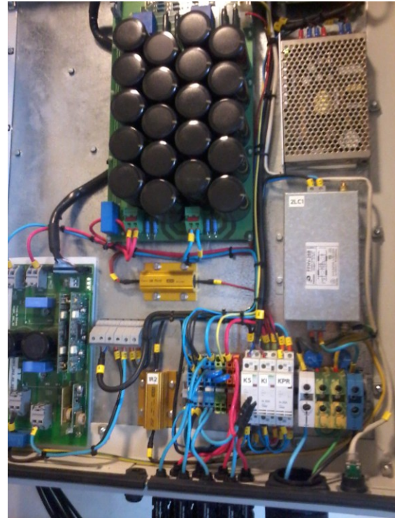
Figure 2. Electronic circuit of the inverter dedicated to the solar photovoltaic generation system installed in the monitoring and control center in Buzios.
