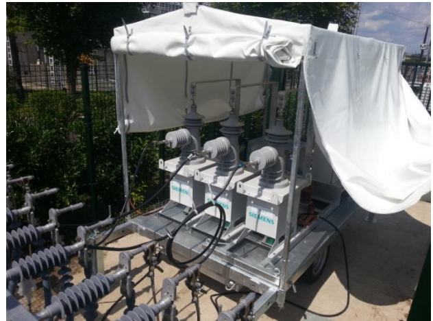
Figure 4. Mobile circuit breaker
