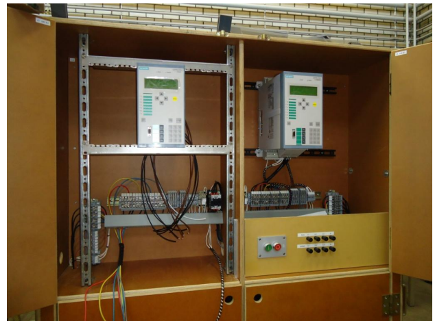
Figure 2. Part of the original hardware simulator
